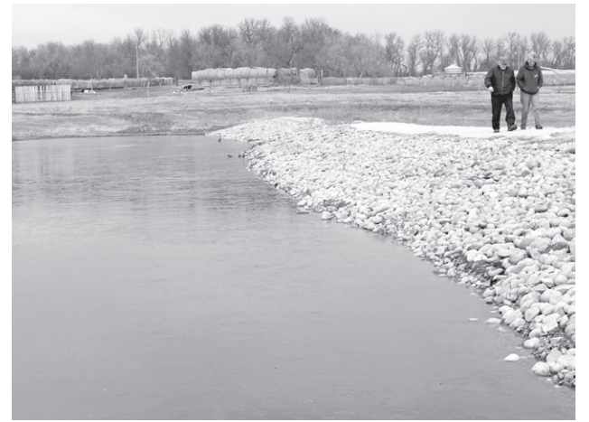
The dam was degraded and DUC did a rebuild in 1983 and again in 2024.
