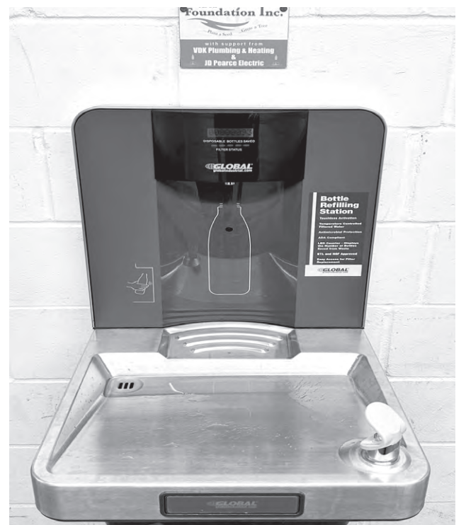
Manitou Community Arena - Water Bottle Filling Station $3,600.00.
